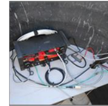
Datalogger within vault
